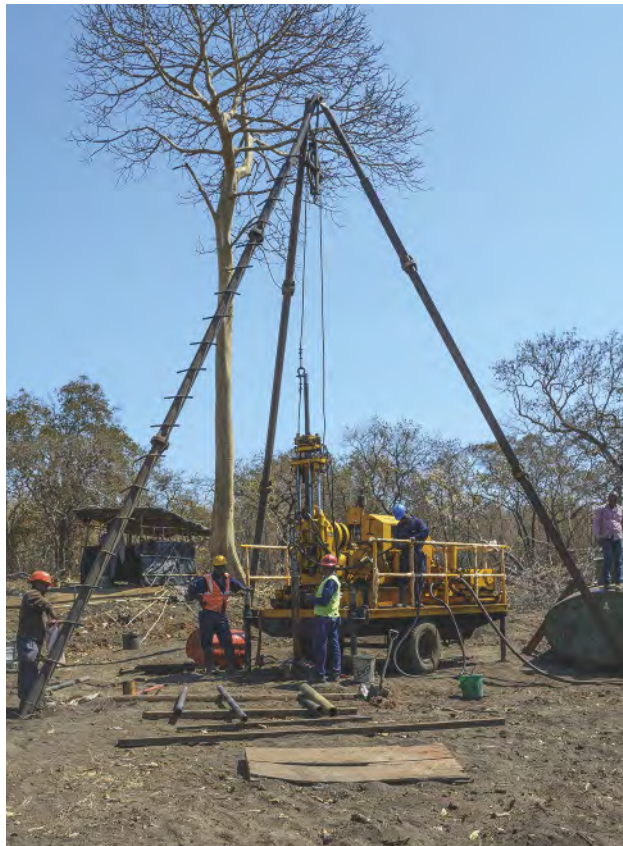
Figure 13. The setup of the core-drilling instrument. Water from a tank next to the working platform is run the whole time to cool the drill bit. Photo by Andrew Lucas/GIA.
