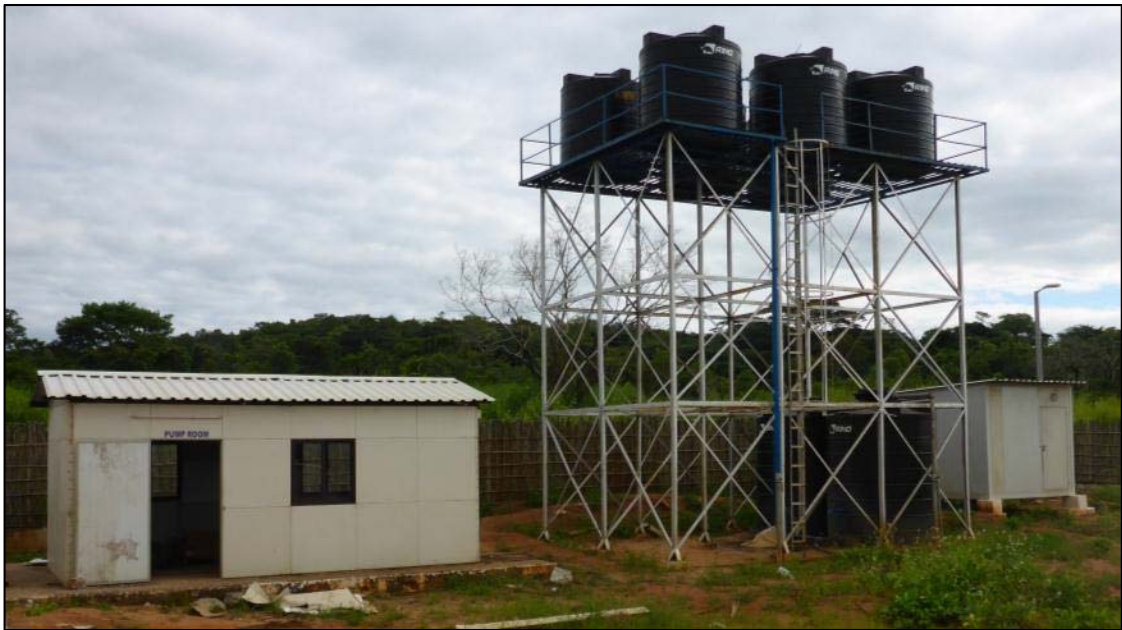
Figure 8-6: Namanhumbir Camp Potable Water Storage Tanks
