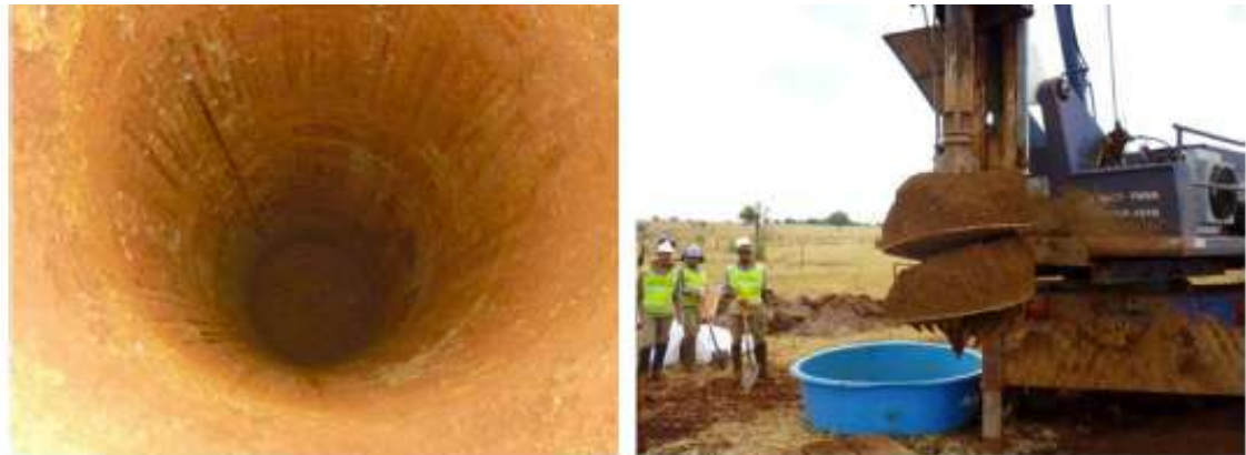
Figure 13.1 1 m diameter auger drill used to take the 130 tonne bulk sample at Pequizeiro in September, 2011
