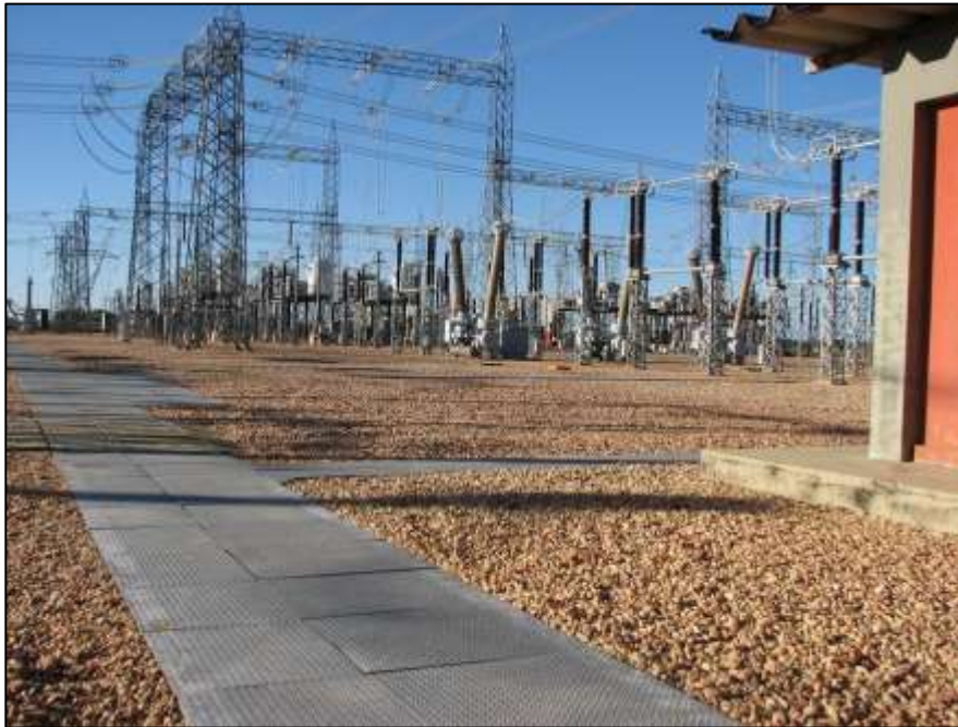
Figure 18.18 Existing Colinas substation
